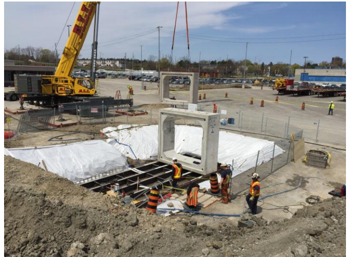
At Guildwood GO Station, the crane lifts precast tunnel sections and places on grillage in preparation for July tunnel slide work.
